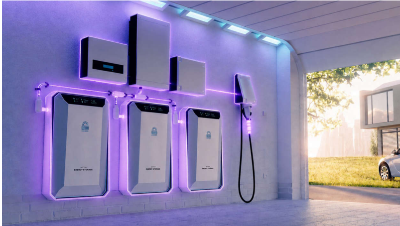
Figure 2. An intelligent monitoring system ensures that bidirectional energy flows seamlessly while protecting the home from faults and hazards
