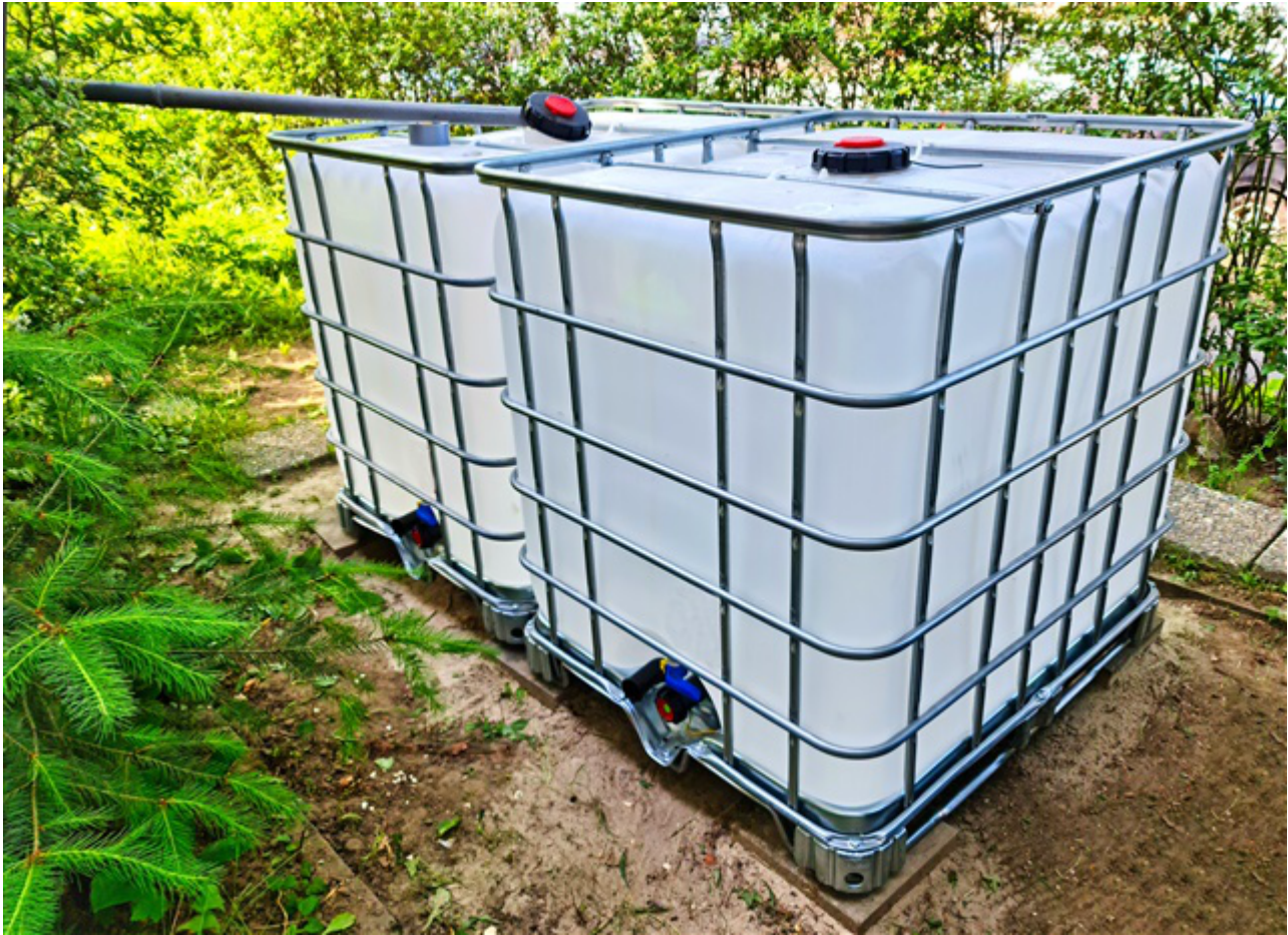
Figure 5. 77GHz radar sensor installed at the top of the Industrial tank for level measurement
